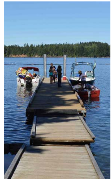
Many of the park activities are focused around lake access. This photo shows dock upgrades in progress.
