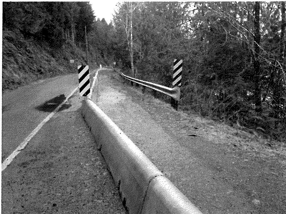
Photo 1 - Eastern end of the Comox Lake Road Shoulder Failure
