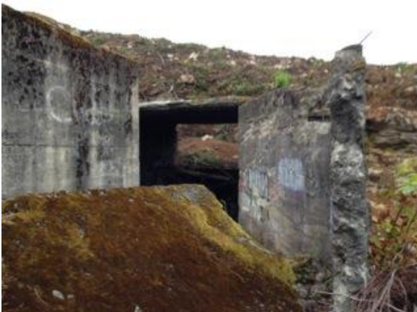
7. Collapsed roof section over south bay
