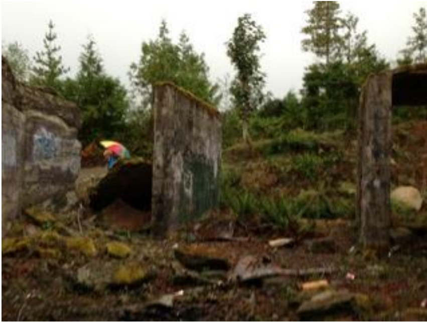
8. Fin walls looking west with collapsed roof slab to left
