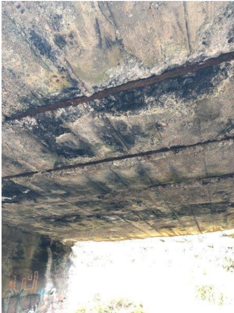
Photo 7 Embedded Steel Channels in Roof Span with Severe Spalling
