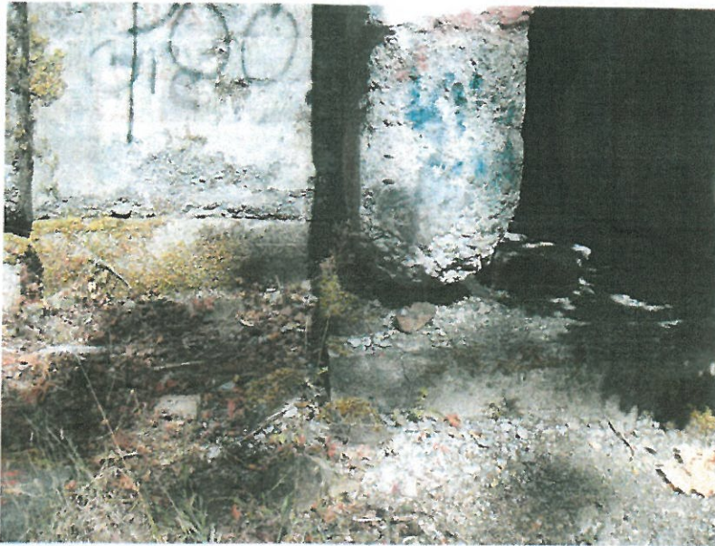
Photo 5 – Entrance Walls eroded at Base
