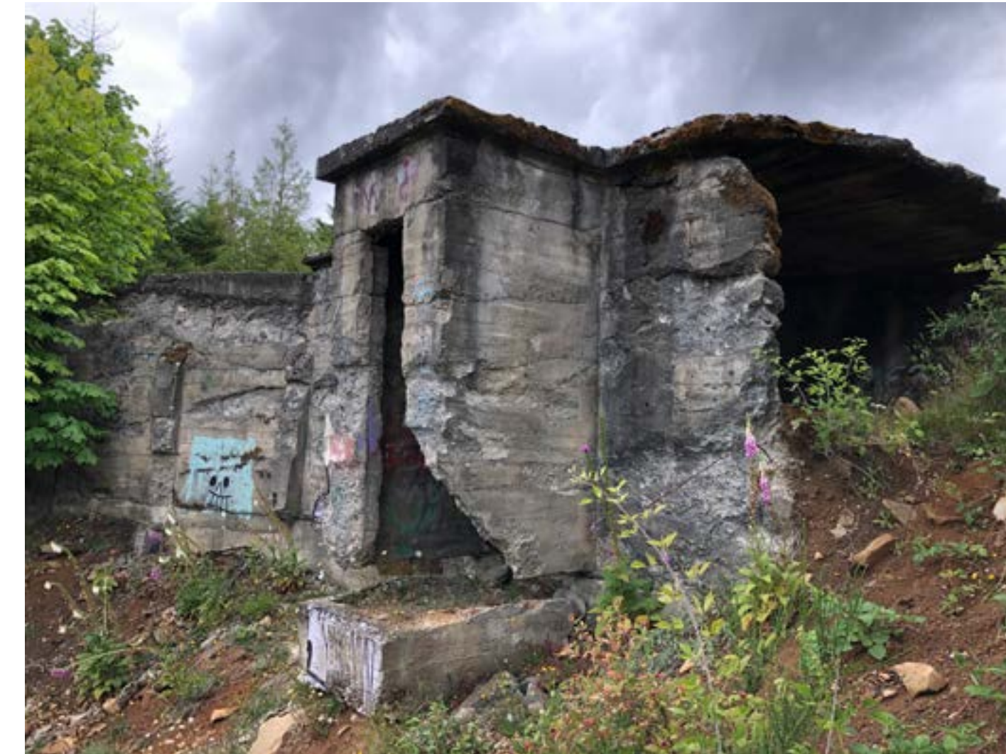
ACCESS DOOR AND VENTING SHAFT
