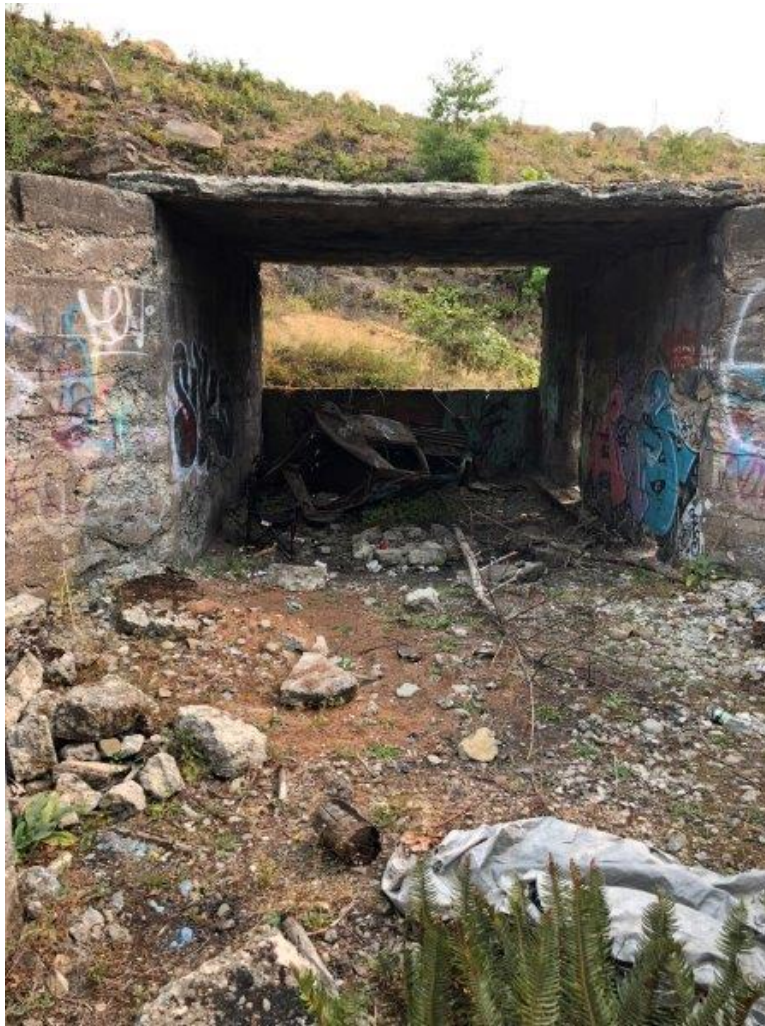
Photo 6 Remaining Roof Span. Note Concrete Deterioration
