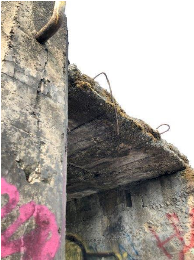
Photo 5 Inadequate Steel Reinforcement in Concrete
