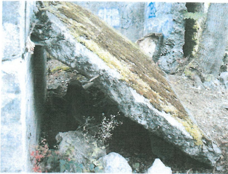
Photo 3 – Fallen Roof Slab Adjacent to Tree
