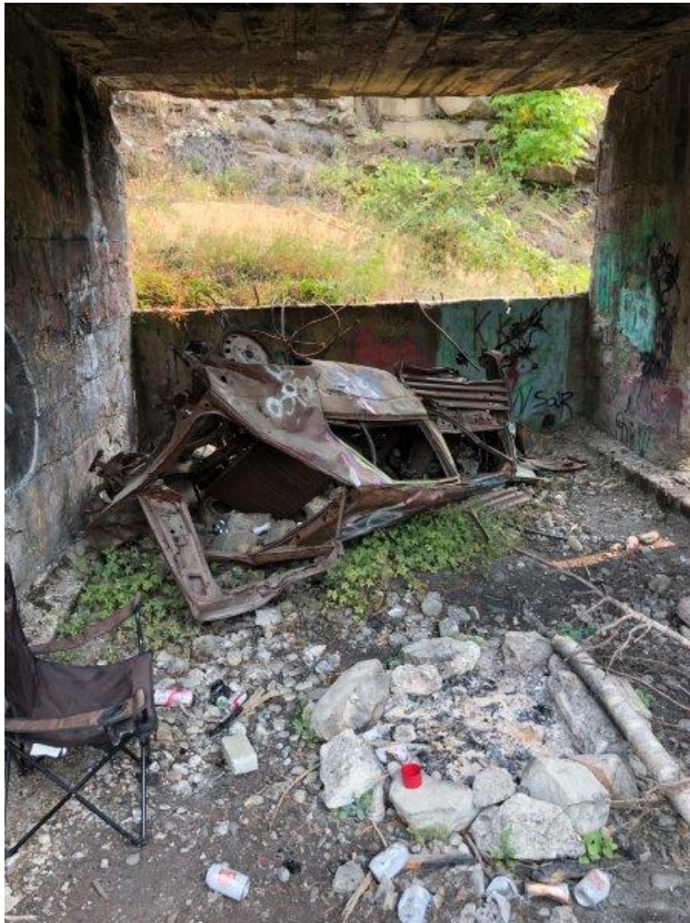
Photo 8 Evidence of Public Accessing the Structure
