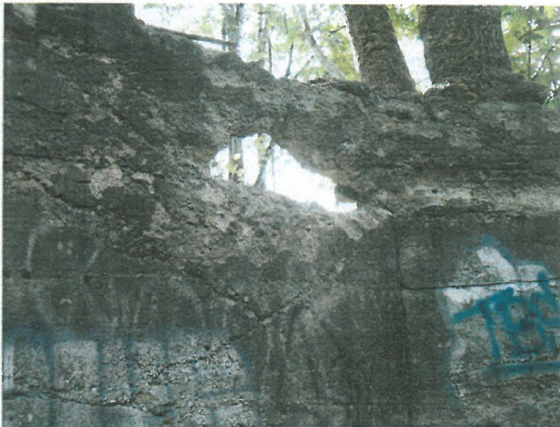
Photo 4 – Holes in Concrete Walls
