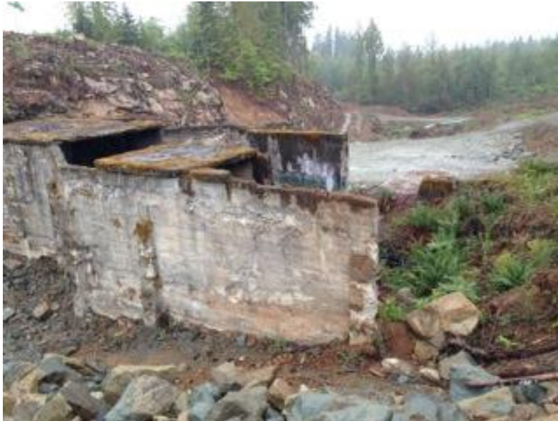
Ruin of reinforced concrete walls
