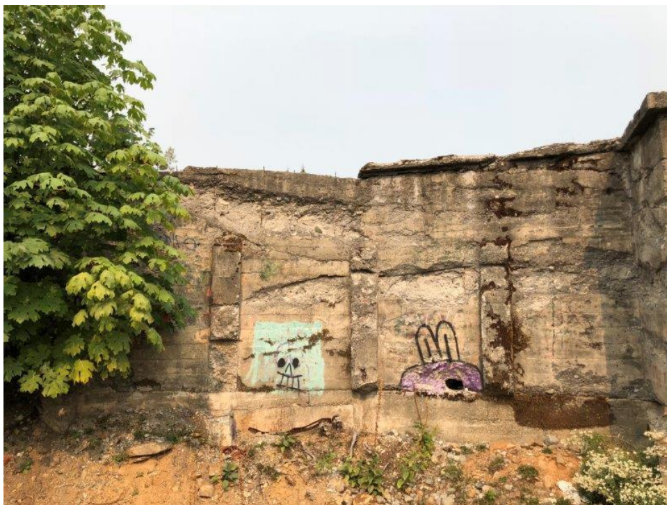
Photo 3 Concrete Walls in Poor Condition. Note Extensive Cracking and Spalling
