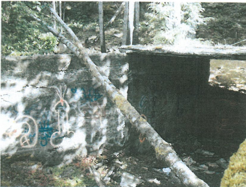
Photo 2 – Center Section of Roof Missing
