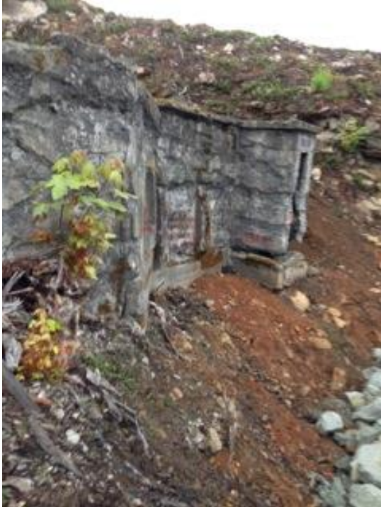
18. Undermining of concrete foundations on south side
