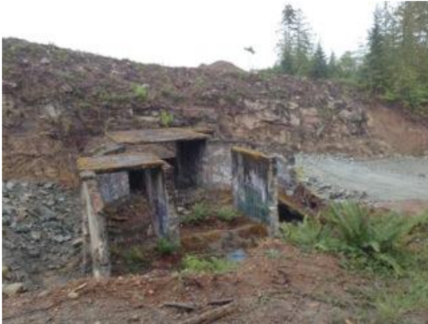
2. View from west across canyon showing concrete fin walls with collapsed wall & roof to the south (right)
