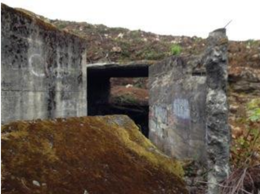
7. Collapsed roof section over south bay
