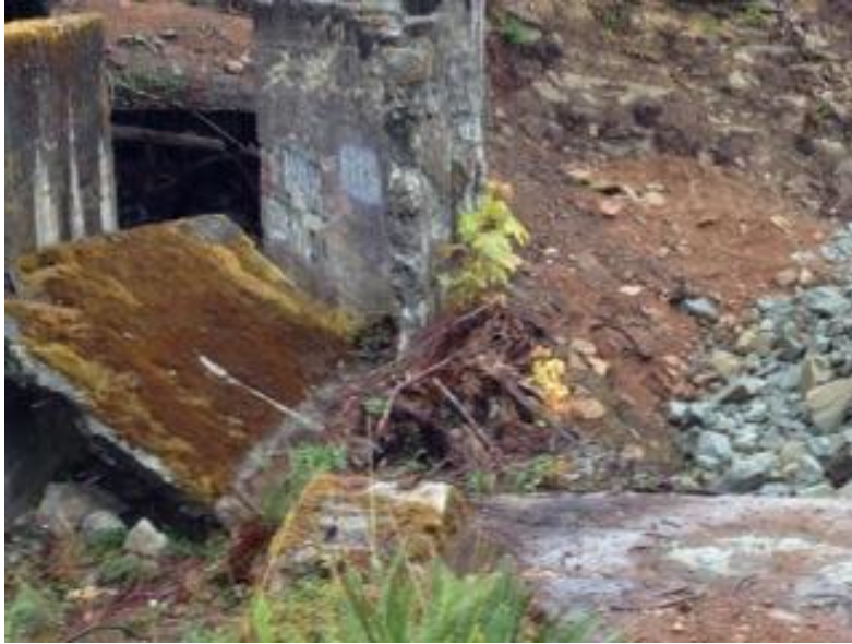
Collapsed roof slab
